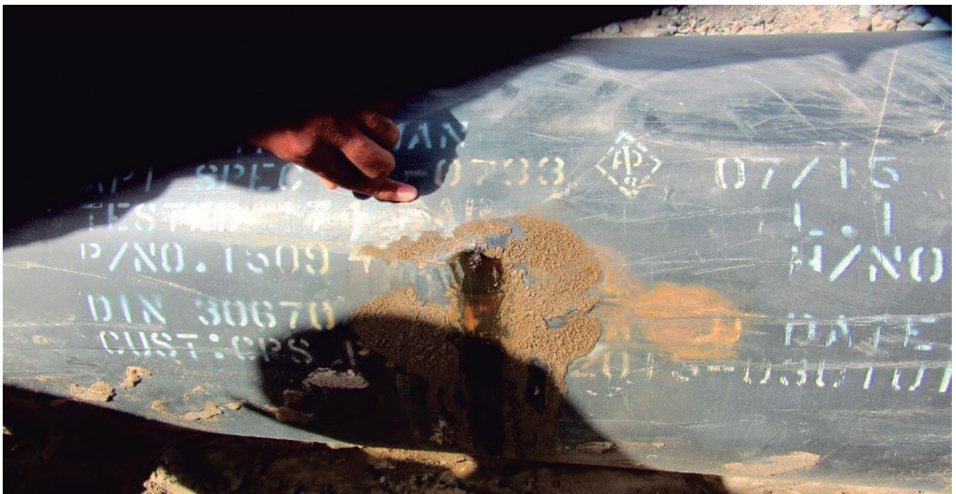
Figure 5: Leak detected on a pipeline in Oman using the Pig Point technique
